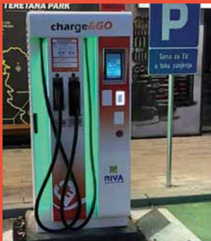
Riva Park Velika Plana 120 kW charger
