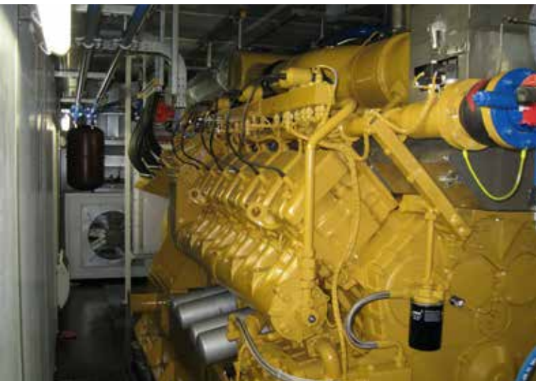
◀ ▲ An example of a realized project -Interior appearance: gas engine
